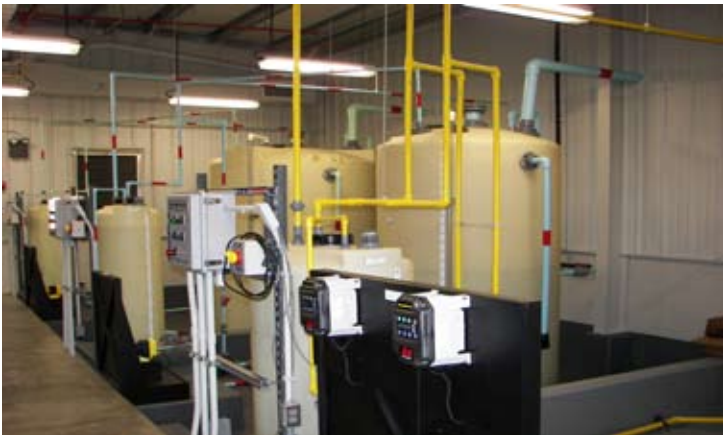
The inside of the new Water Works Chemical Feed building, the tanks, pumps and piping
